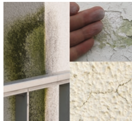
ALGAE, FUNGI, CHALKING, BLISTERING OR CRACKING ARE JUST A FEW EXAMPLES OF FACADE DESTRUCTION.
